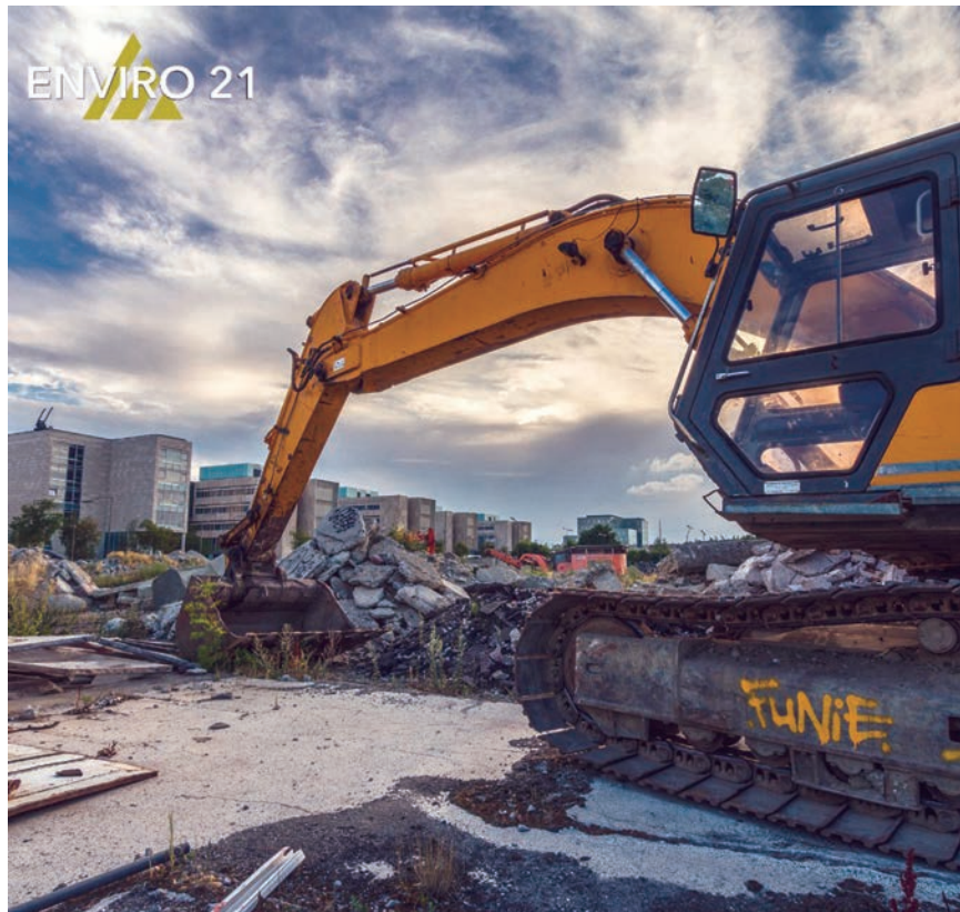
Enviro 21's expertise in the demolition and waste industry helped construct a bid that ensured the city would pay no extra costs, while complying with all laws and regulations. Photo courtesy of Enviro 21.
